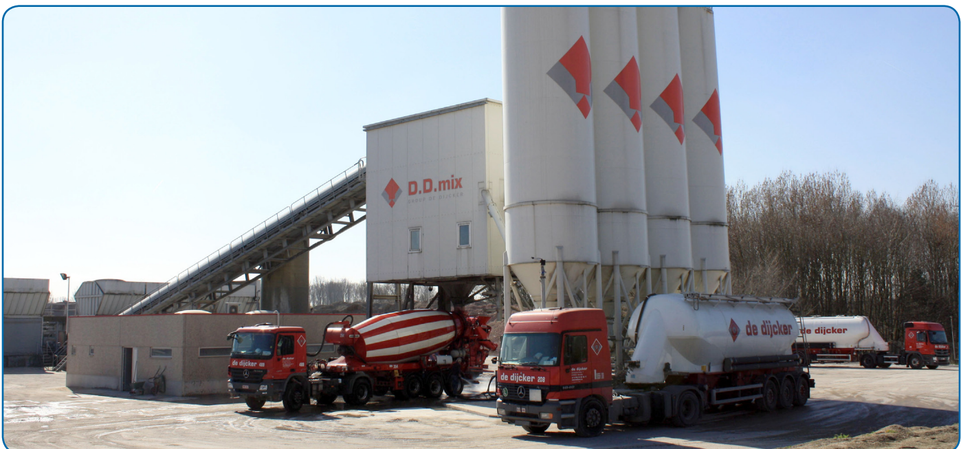
One of the D.D. Mix concrete plants owned by De Dijcker NV.
