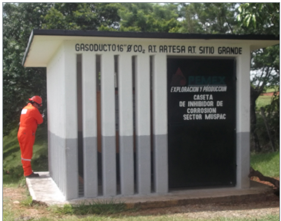
In some areas, the oil company plans to protect Neptune’s pipeline corrosion-injection systems with enclosures designed to keep out the elements and eliminate instances of tampering.
